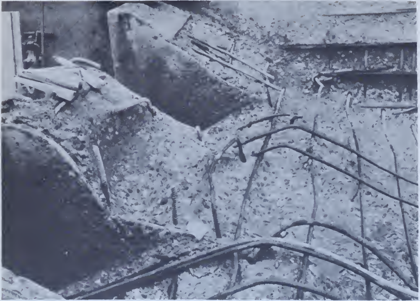
Figure 7. —Abrasion erosion of concrete in the dentates, walls, and floor of the Yellowtail Afterbay Dam sluiceway stilling basin. The “ball-mill” action of cobbles, gravel, and sand in turbulent water abraded the concrete, thus destroying the integrity of the structure. P459-D-68905.
